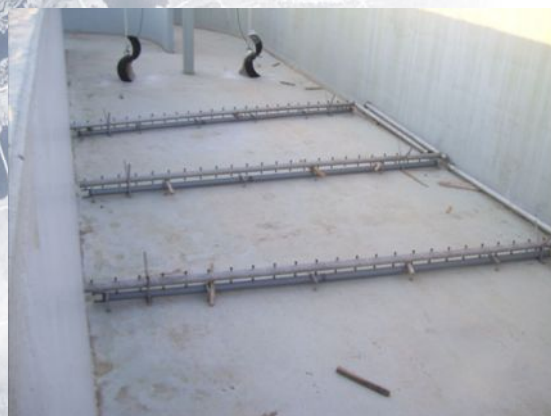
Air Piping and Flow Boosters in Bio tank
