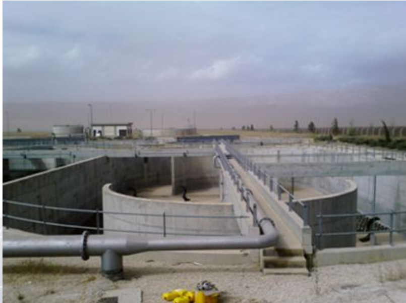
General View of The Bio Tank
